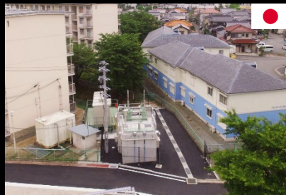
Kyoguchi Pumping Station 700mm / 1.05cms / 2.6mH / 2units
