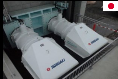
Kamikawa Pumping Station 1200mm / 3cms / 2.9mH / 2units
