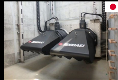
Futago Pumping Station 1000mm / 2.13cms / 3.1mH / 2units
