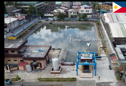
Balut Pumping Station 1200mm / 3cms / 3.3mH / 1unit
